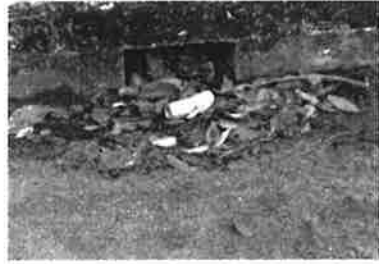
(c) clogged inlet
